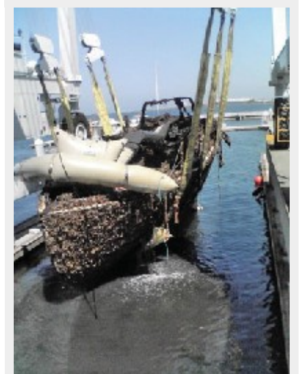
Beyond 'Wreck'ognition - Vessel Assist in San Diego was contracted recently to remove wreckage beneath A-8 Anchorage. Originally asked by the Port of San Diego to cleanup a dozen wreck sites, the project was scaled back to half that number after the port realized the magnitude of some of the wrecks.
